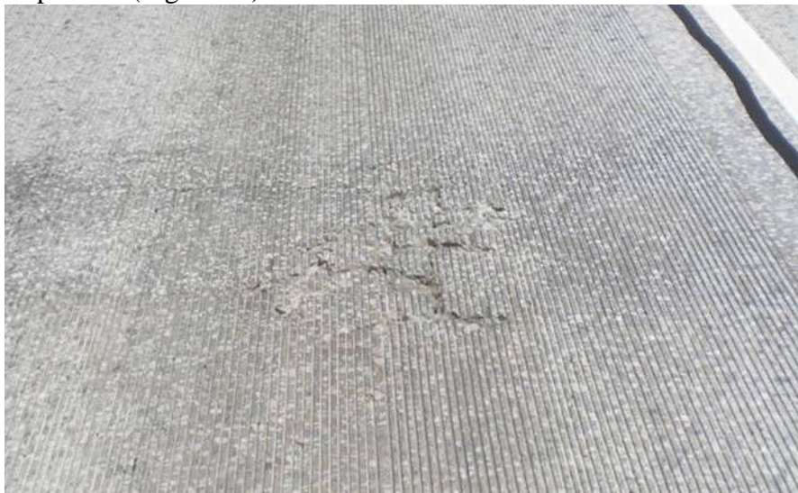
Figure 15. New Material Failure on Quiet Concrete Demonstration Projects – SR 76, Richmond.
